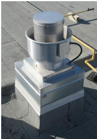
Figure 6: Kitchen Roof-mount Exhaust Fan
