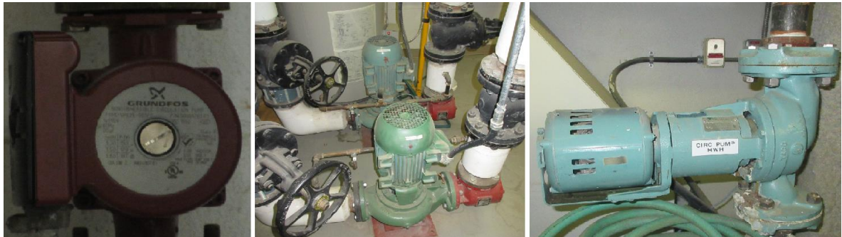
Figure 7: DHW Recirculation Pump (Left), Boiler Hot Water Pump (Center), Hot Water Circulation Pump to MUA-3 (Right)
