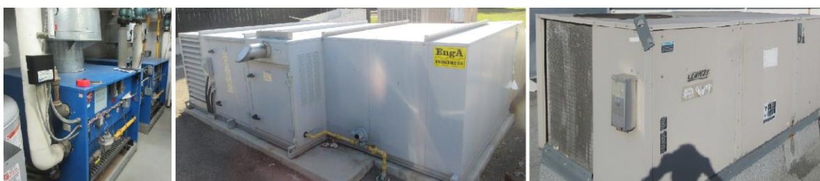
Figure 3: Boilers (Left), MUA (Center), RTU (Right)
